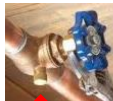
Shutoff valve with drain
