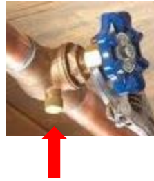
Shutoff valve with drain
